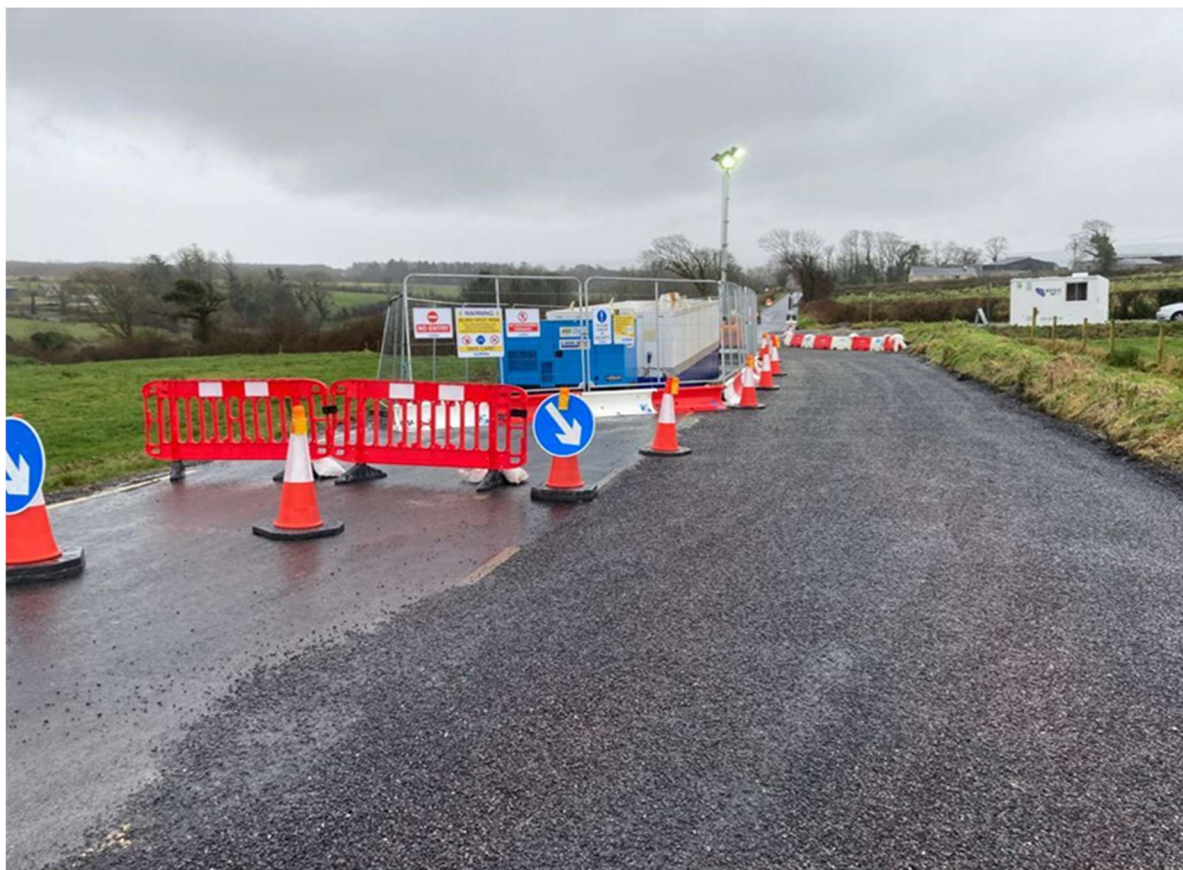
Image 1.5: Example of a Passing Bay (Ensuring Road Traffic Continues Around a Working Area)
