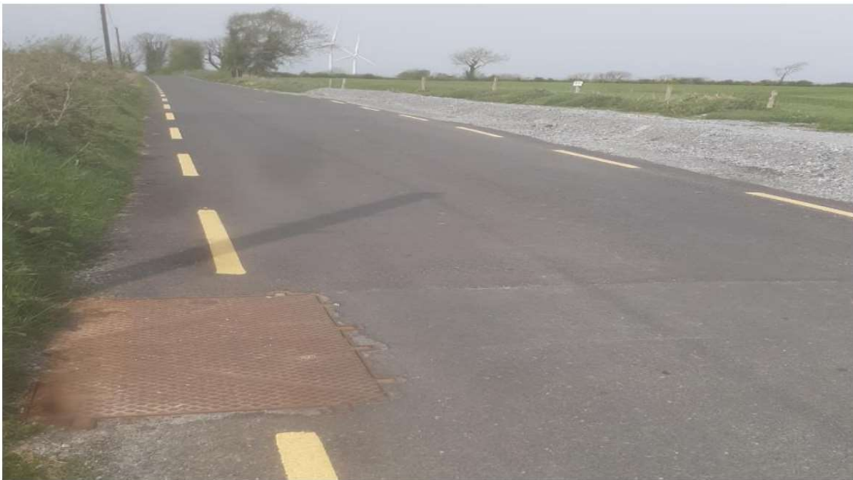
Image 1.4: Example of a Reinstated Road Over a Joint Bay (Darker Asphalt) with the C2 Chamber Cover Visible
